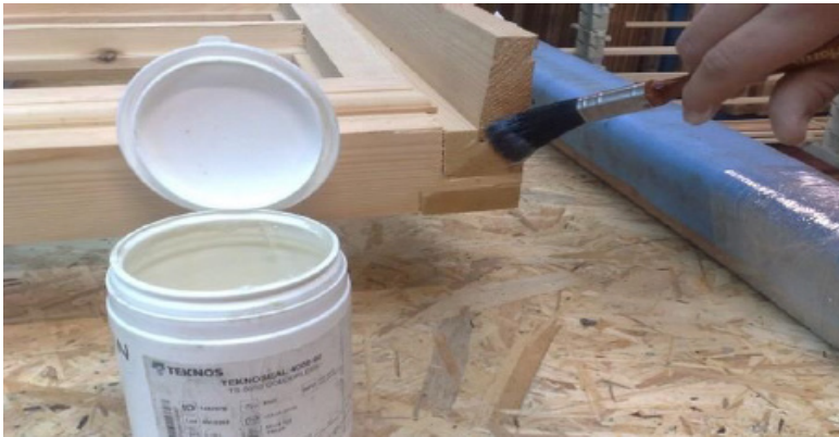
TEKNOSEAL 4000 applied by brush to exposed end grain after applying Combi Primer 2907.
