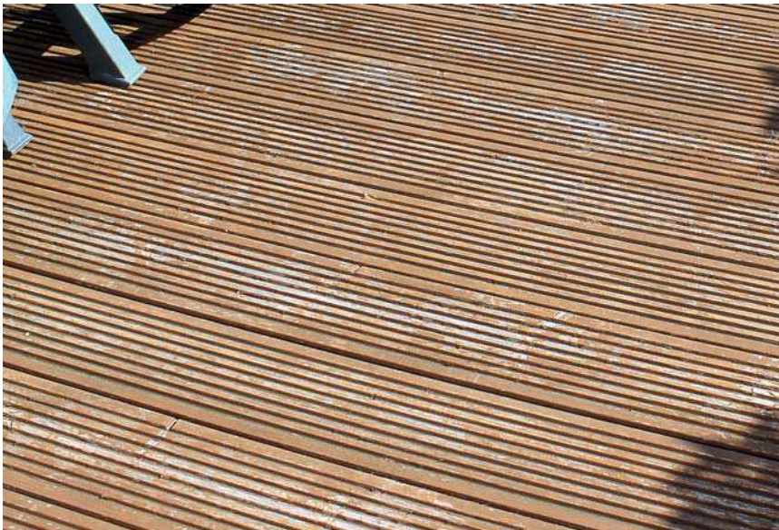
Above shows the extent of the problem on one area of decking
