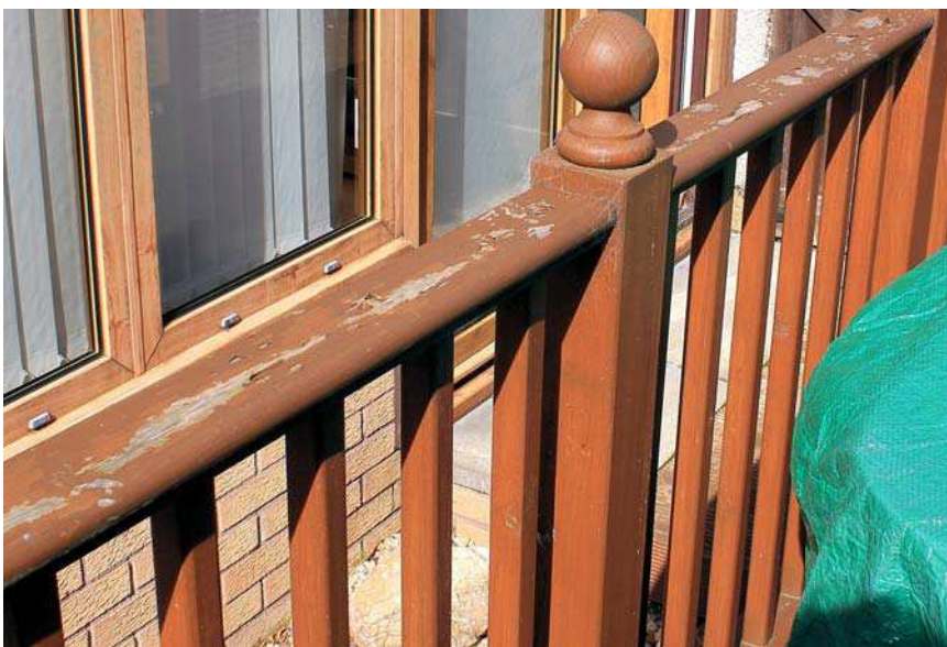
Above shows the extent of the problem on two areas of handrail
