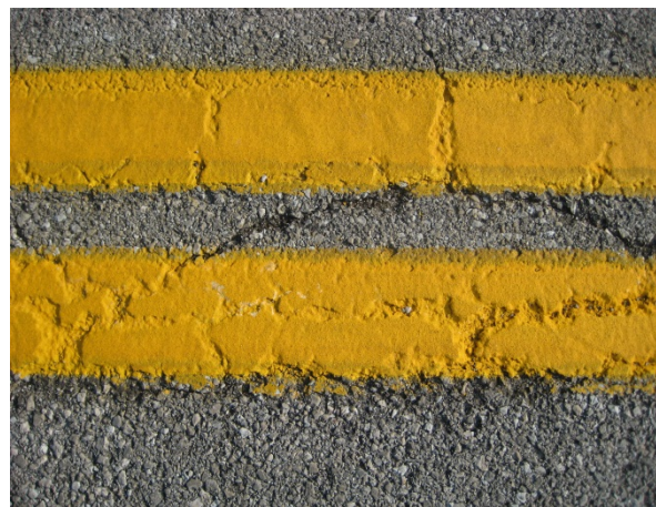
Low Reflectivity Numbers: Overlapping layers of paint are built up beyond acceptable limits. Should be removed prior to new paint application.
