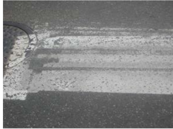
Paint Discoloration/ Tire Tracks on Paint: Highway traffic paint used on parking lot. This type of paint is to be installed using glass beads.
