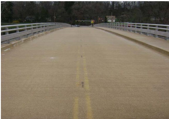
Paint Bonding Failure on Concrete: Concrete curing compounds not removed from bridge deck prior to application.
