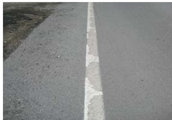
Paint Bonding Failure on Asphalt: Surface not properly cleaned prior to application.
