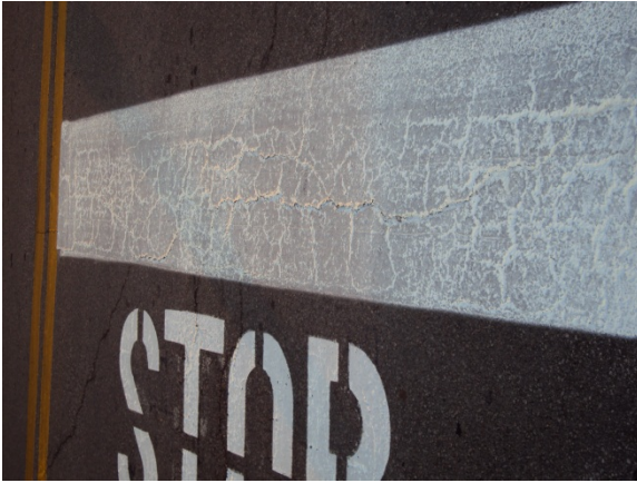
Paint Bonding Failure: Surface not properly cleaned prior to installation. Not properly cleaned between multiple passes.
